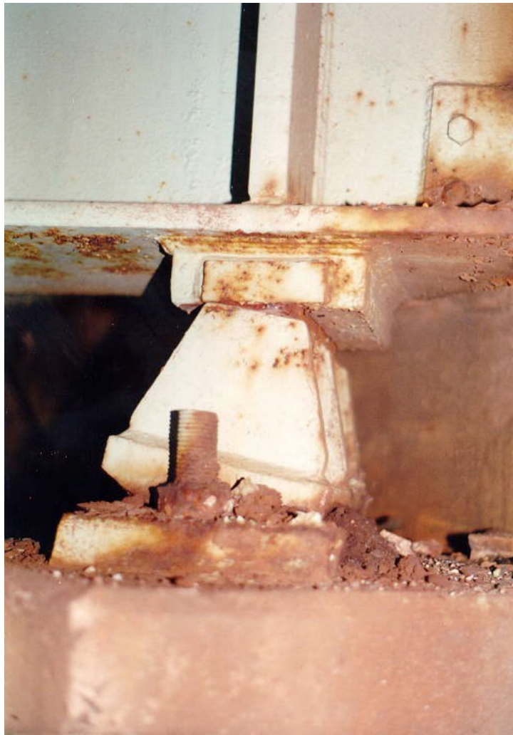
Figure 5.7.1-9 Over Extended Rocker Bearing.
