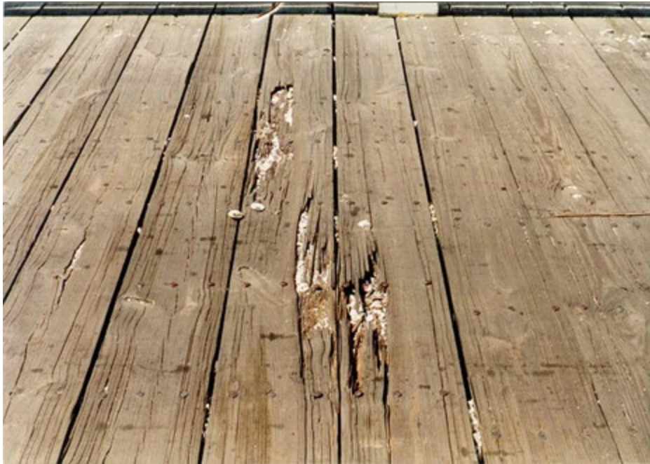
Figure 5.6.1-1 Deterioration of timber plank deck surface.
