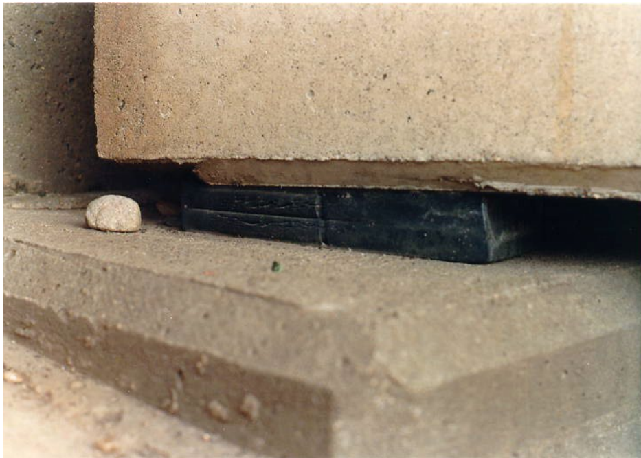
Figure 5.7.1-13 Elastomeric Bearing. Note the Non-parallel Bearing Surfaces Causing Bulging and Cracking at the Rear of the Elastomeric Bearing Pad.
