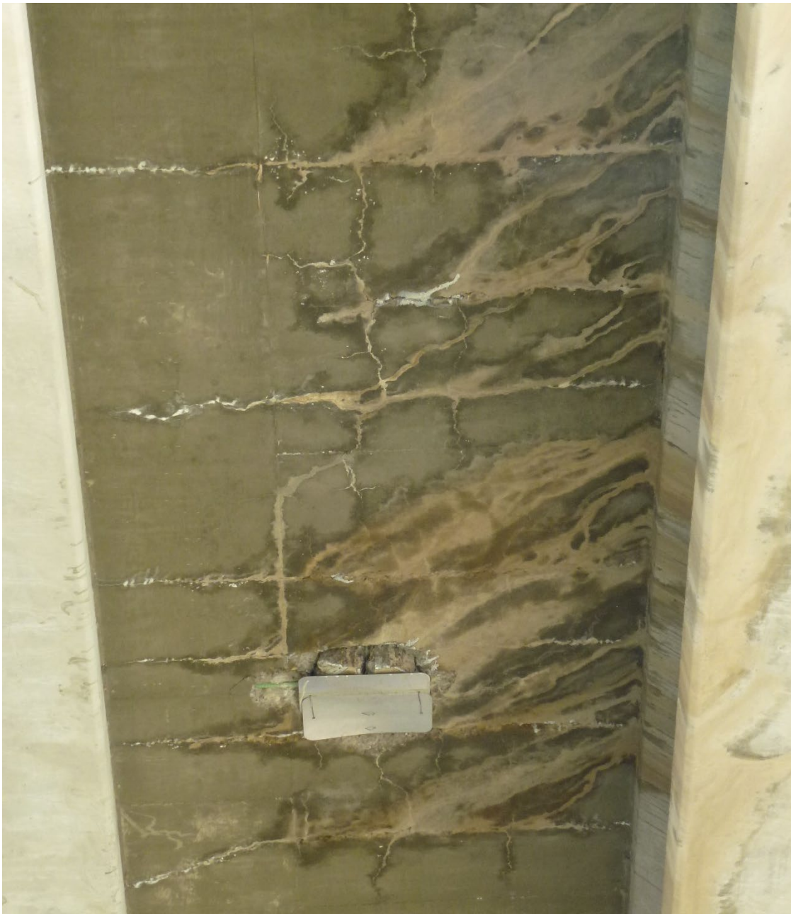
Figure 12. Example of Condition State 4. Tight spacing, jump cracks, “islands”, grey colored efflorescence present, very heavy water staining, repaired hole
