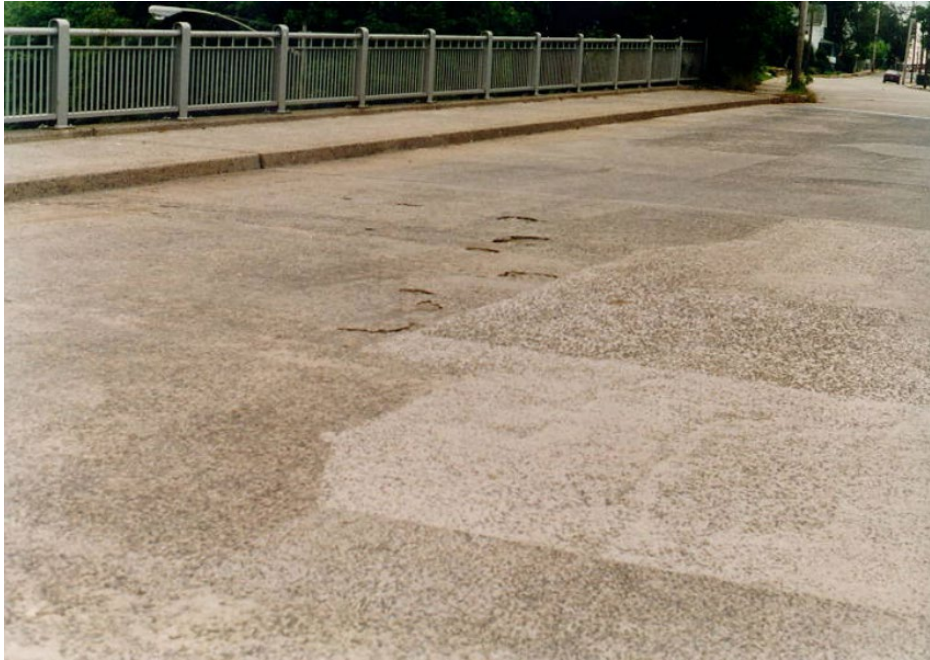
Figure 5.6.2-1 Top of Bare Concrete Deck with Patched, Spalled and Hollow Areas.
