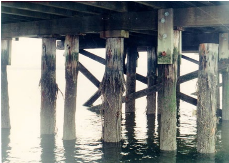
Figure 5.8.3-1 Timber Pile Bent exhibiting Freeze-Thaw Damage above the waterline. Also examples of shims, blocking and splices between the piles and pile cap
