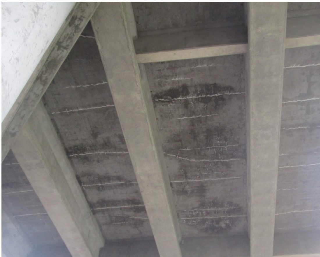
Figure 3. Typical Transverse Cracks Seen from Underneath
