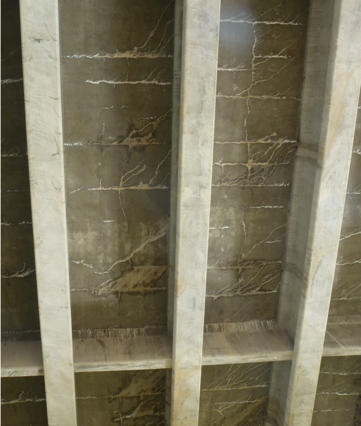
Figure 11. Example of Condition State 4. Note the tight spacing, multiple jump cracks (some creating the concrete “islands”), very heavy gray staining and efflorescence.
