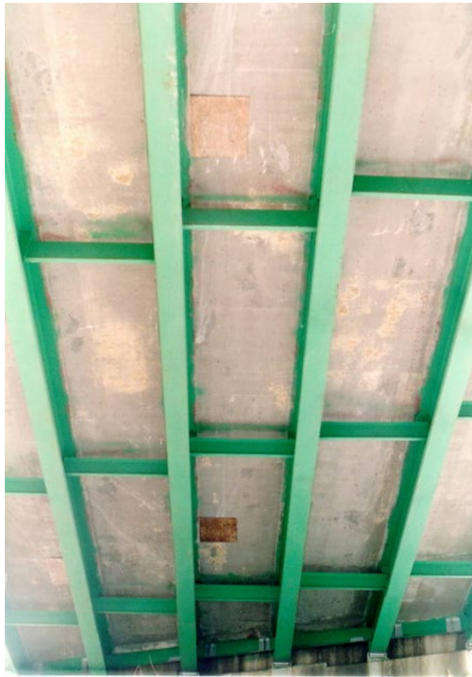
Figure 5.6.2-2 Typical Underside of Concrete Deck. Note Cracking with Efflorescence and Formwork Remaining from Full Depth Patching.
