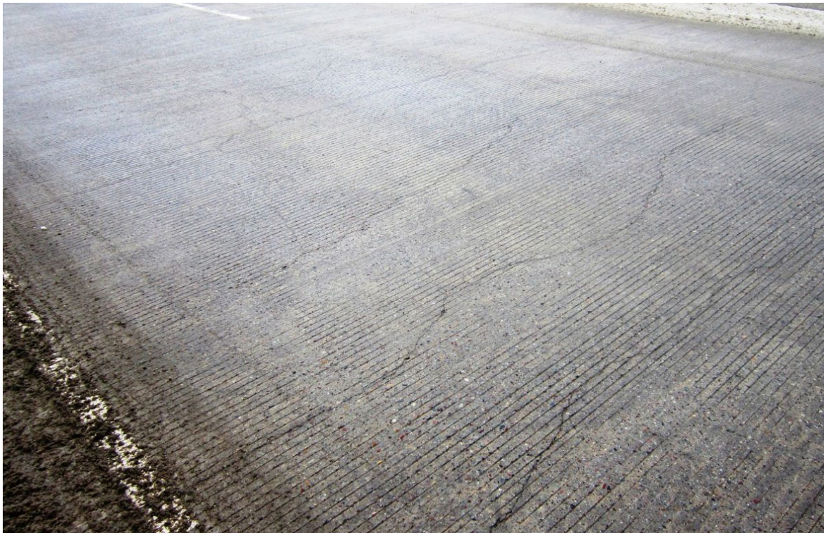
Figure 2. Transverse Cracks in Bridge Deck
