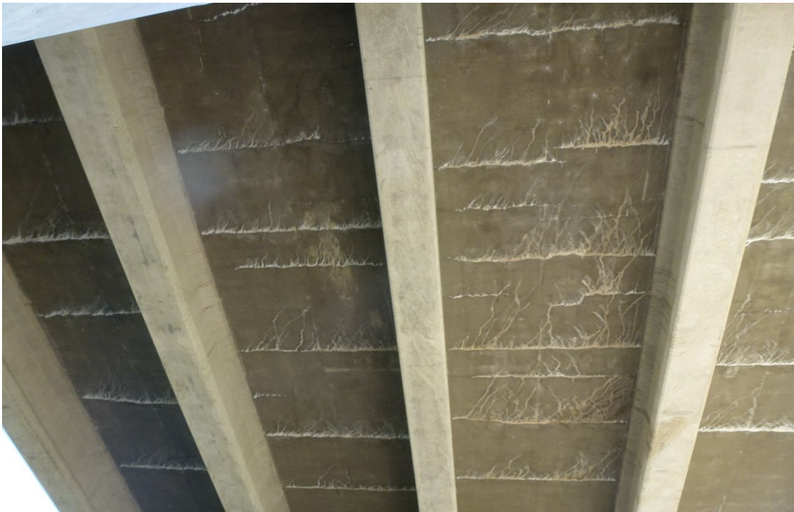
Figure 9. Example of Condition State 3. Note the tight spacing (12” to 18”) of some of the transverse cracks, along with evidence of heavy leakage and some gray efflorescence. Also, small jump cracks evident.
