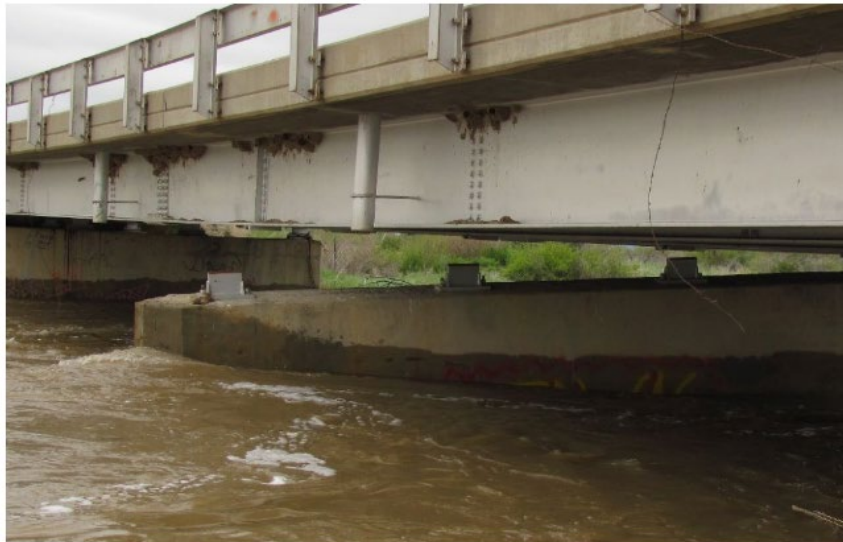
Figure 5.9.2-1 Pier Settlement due to Undermining
