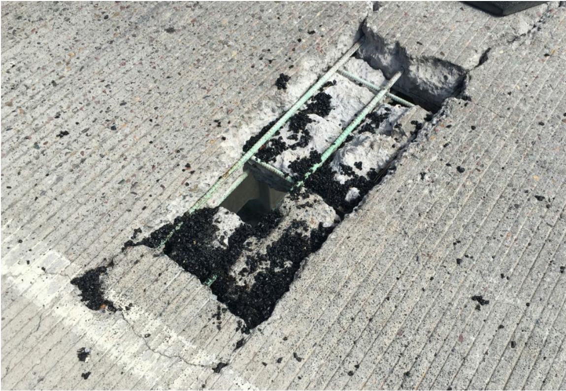
Figure 4 – Holes in Bridge Deck. Note the longitudinal jump cracks that create the rectangular “island” of concrete. The “island” continued to crack until full depth chunk or “island” fell out, creating the hole.
