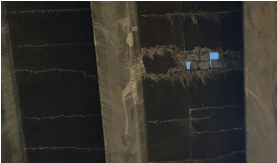
Figure 5. Same hole as Fig. 4 as seen from Underneath. Note the heavy staining on the soffit and girders from leakage in the cracks around the hole and in nearby transverse cracks. Note, little or no staining in cracks in adjacent girder bay. Note jump cracks with beginning staining at another location not far from the hole.
