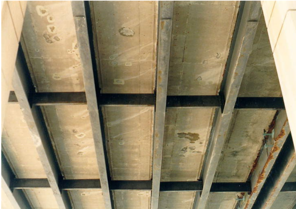
Figure 5.7.8-1 – Typical Rolled Multi-Stringer Superstructure with Ends of Partial Length Welded Cover Plates Visible.
