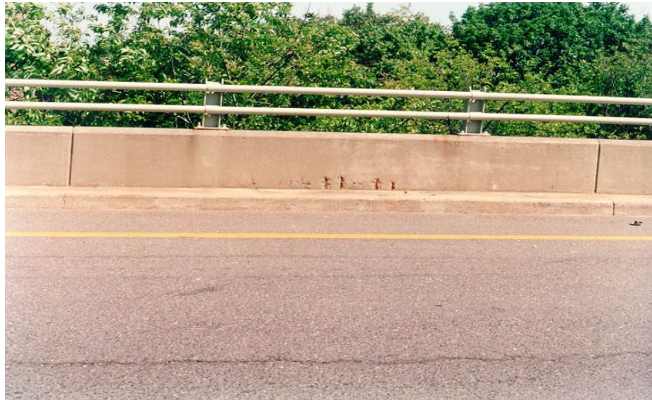
Figure 5.6.8-1 Concrete Parapet with Metal Pipe Railing. Note Spalling with Exposed Reinforcing Steel.
