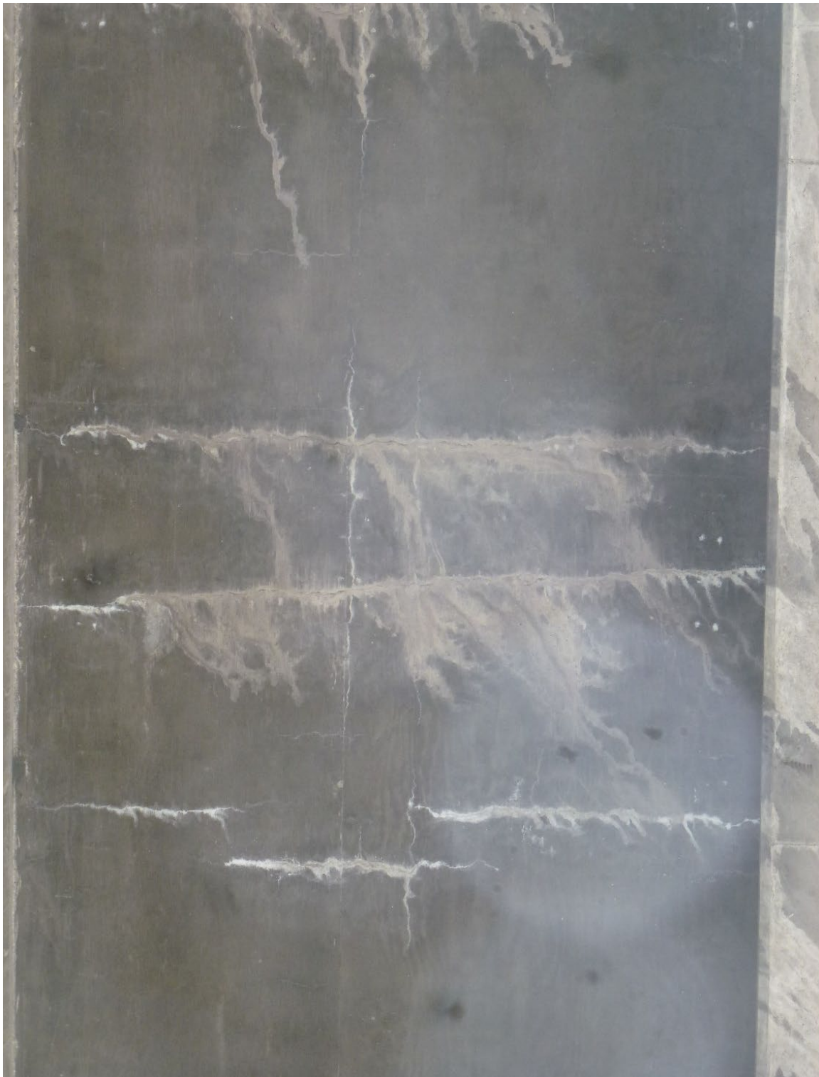
Figure 6. Example of Heavy staining from water leakage. Note the contrast between the gray efflorescence in the upper 2 transverse cracks (evidence of concrete movement around crack and heavy water leakage) and the white efflorescence in the bottom transverse cracks. Note the longitudinal jump crack with light white efflorescence.
