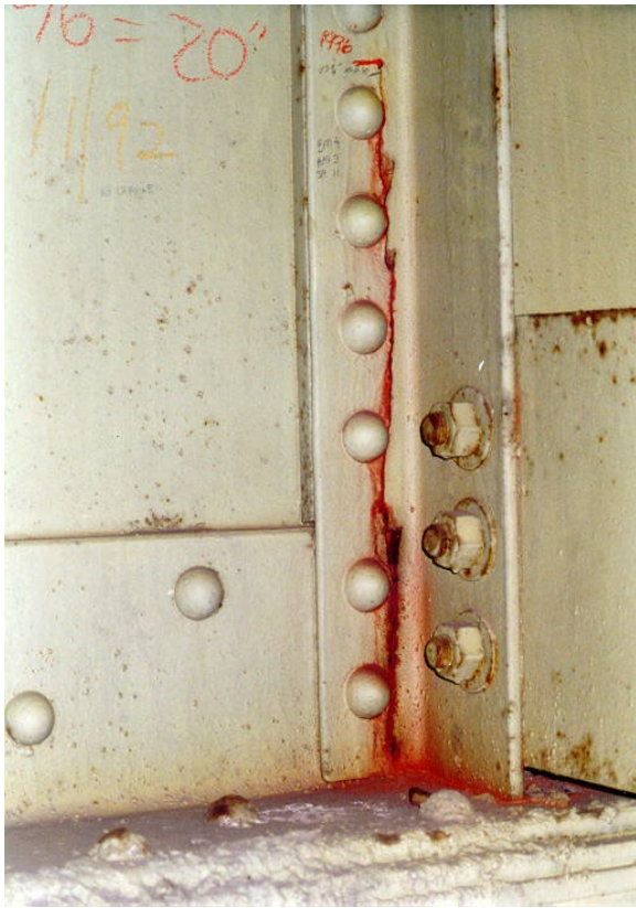
Figure 5.7.8-2 Fatigue Crack in a Diaphragm Connection Angle on a Girder.
