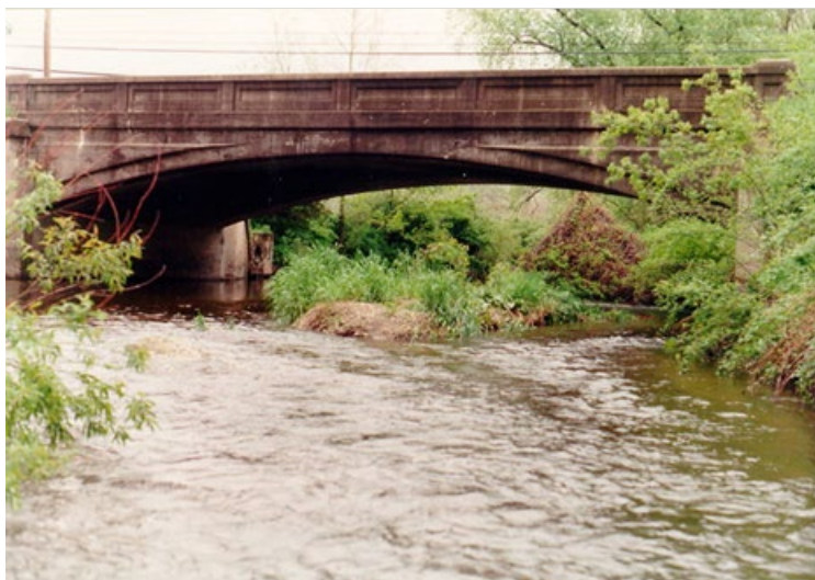
Figure 5.9.1-2 Sand Bar and Vegetation Growth in the Channel.
