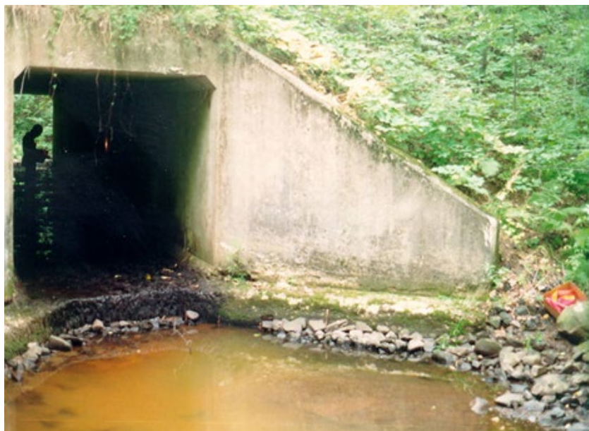
Figure 5.10.3-1 Cast-In-Place Concrete Culvert with Erosion at the Outlet.
