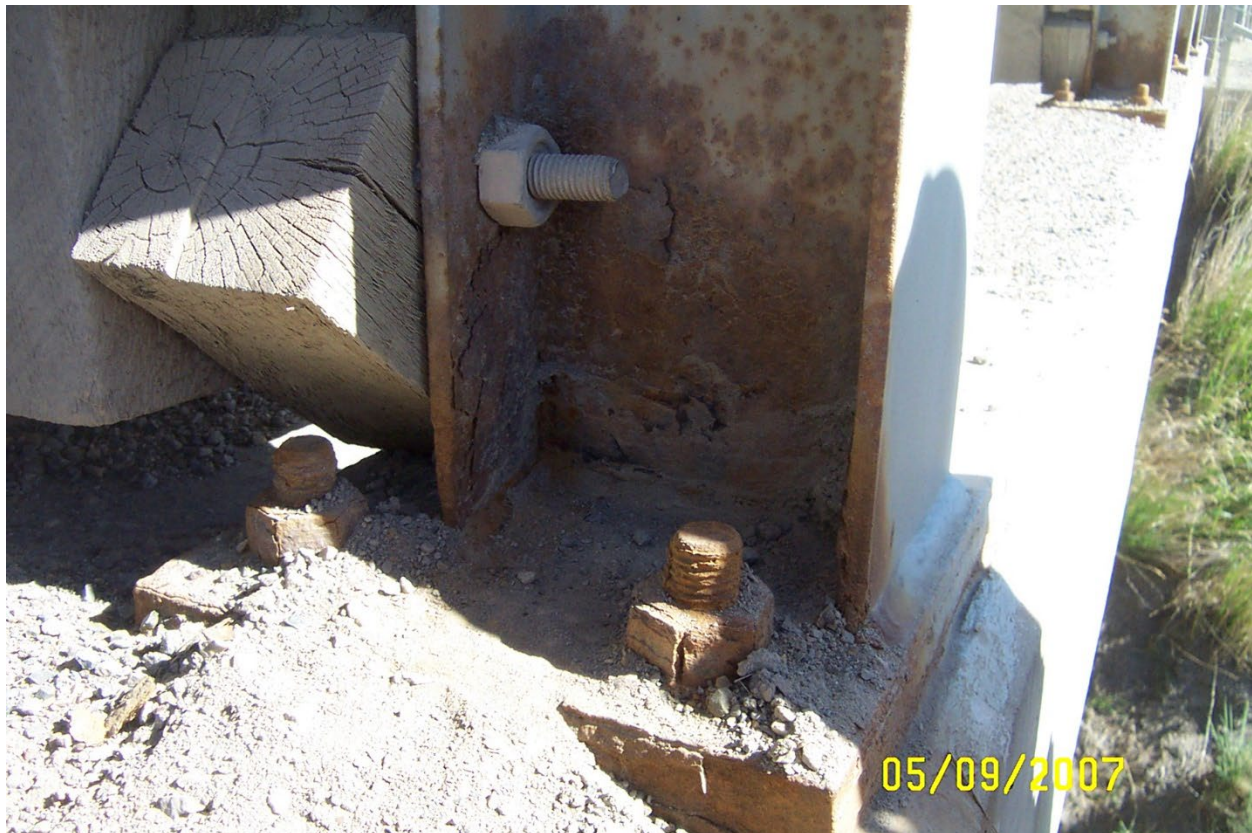
Figure 3.2.9-1 Steel Bridge Railing Post with Corrosion
