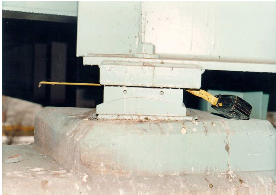
Figure 5.7.1-10 Bronze Sliding Plate Bearing with a Gap Between the Sole Plate and the Sliding Plate.
