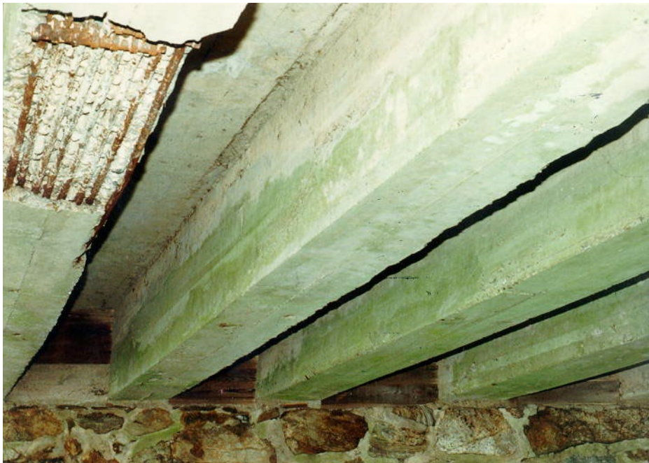
Figure 5.7.4-1 Concrete T-Beams with Large Spalls Exposing the Bottom Layer of Reinforcing Steel
