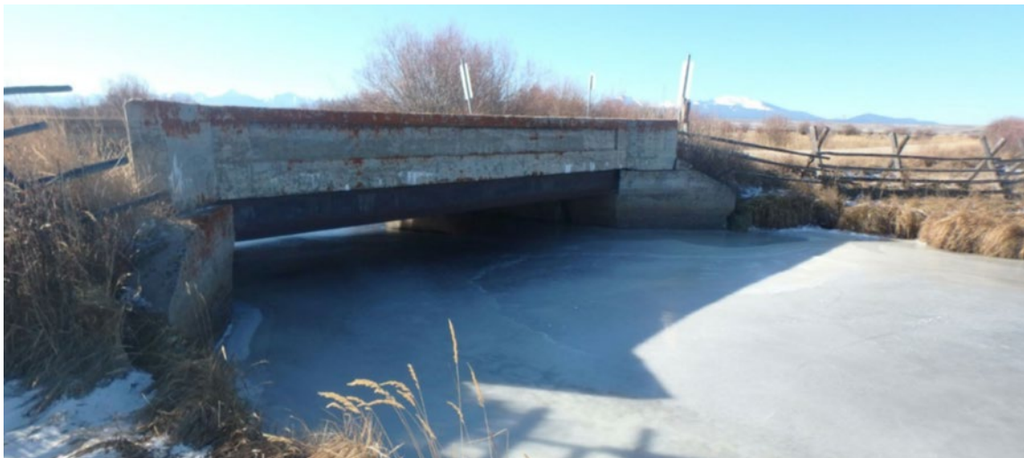
Figure 4.1.8-3 A follow-up inspection is required to check the condition of the bottom of the abutments and to check for scour.
