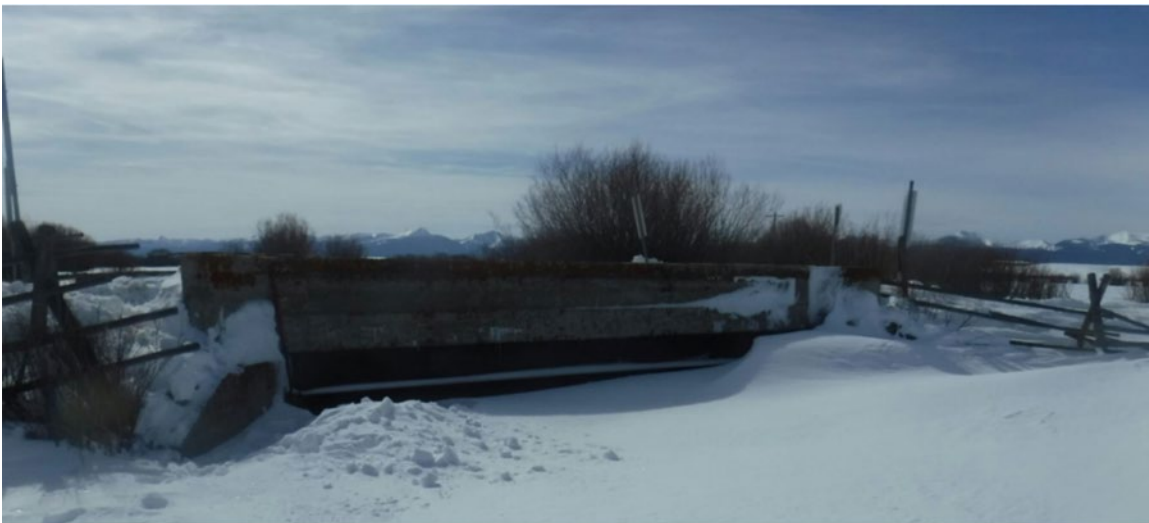
Figure 4.1.8-2 A follow-up inspection is required to check the condition of the wingwalls, abutments, and part of the exterior girder.
