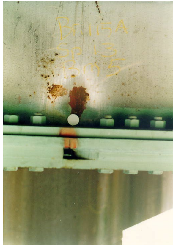
Figure 5.7.8-3 Fatigue Crack Through the Bottom Flange of a Rolled Stringer at the End of a Partial Length Welded Cover Plate. A Stop Hole Has Been Drilled in the Web and Splice Plates Have Been Bolted to the Bottom Flange
