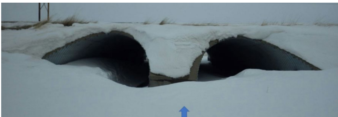
Figure 4.1.8-4 A follow-up inspection is required to check the condition of the pipe culverts.
