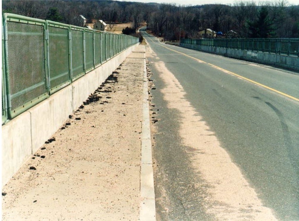
Figure 5.6.9-2 Pedestrian Fence atop Concrete Parapet.
