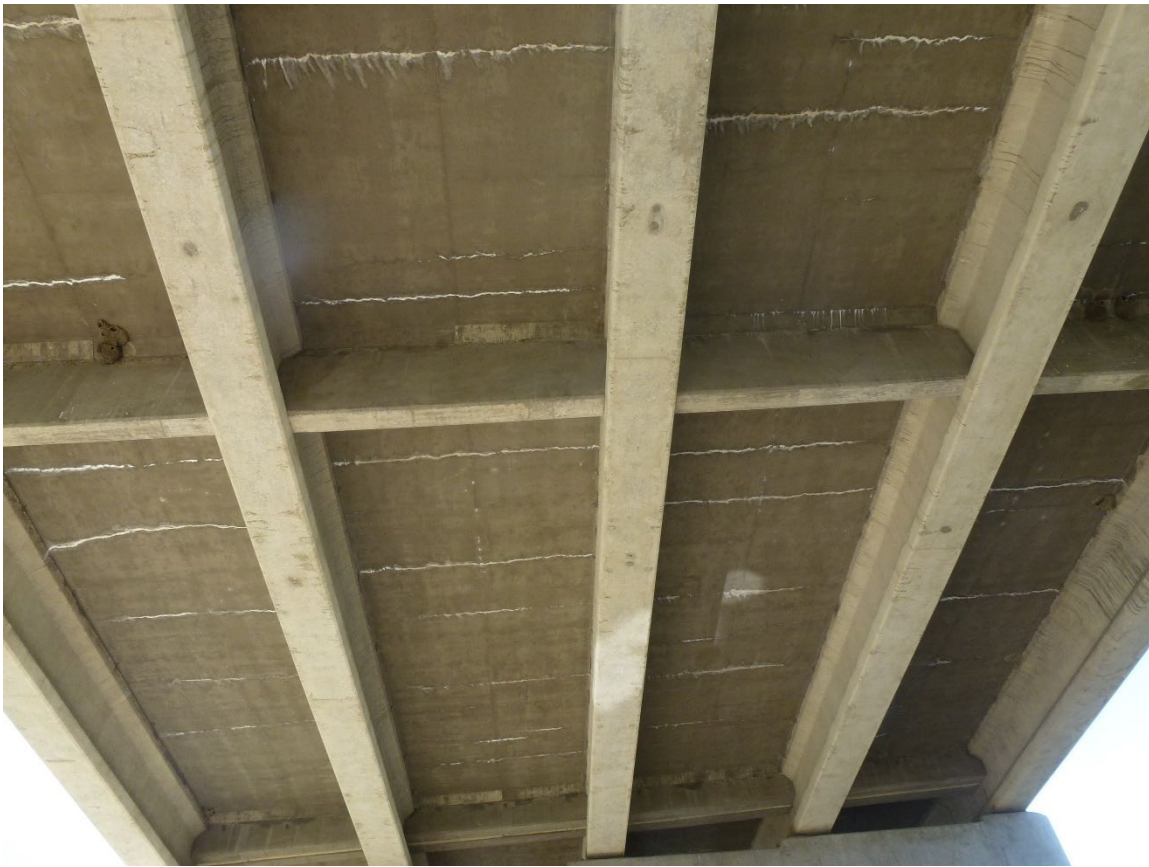
Figure 7. When to not use jump cracking defect. Use the deck cracking defect only. Transverse cracking is present but sporadic. Note the wide crack spacing, the lack of staining, and no longitudinal jump cracks. All efflorescence is white.
