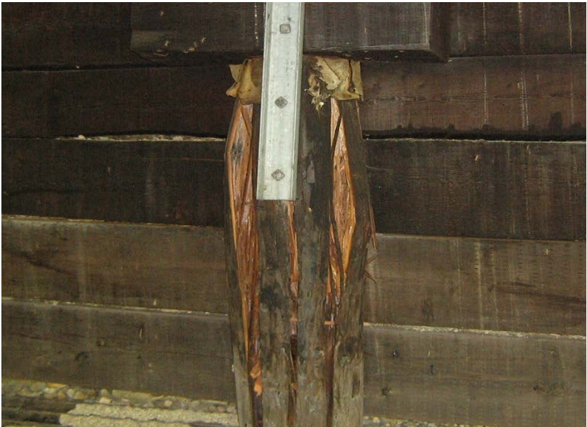
Failed timber pile
