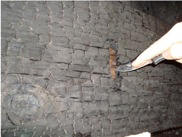
Burned timber members with the char layer scraped off
