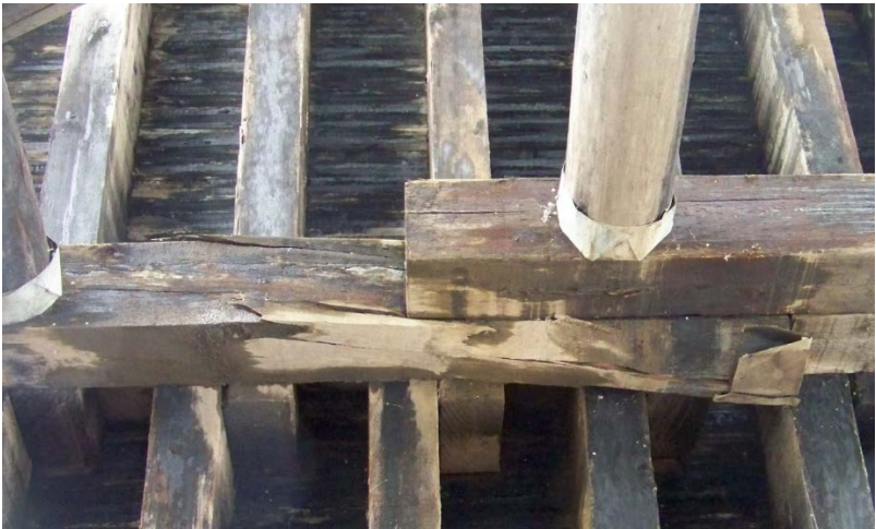
Severe crushing due to decay
