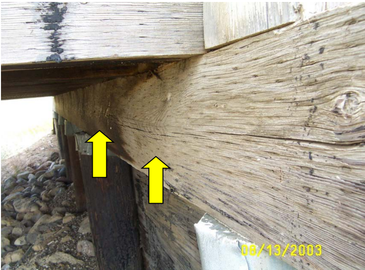
Bulging due to decay
