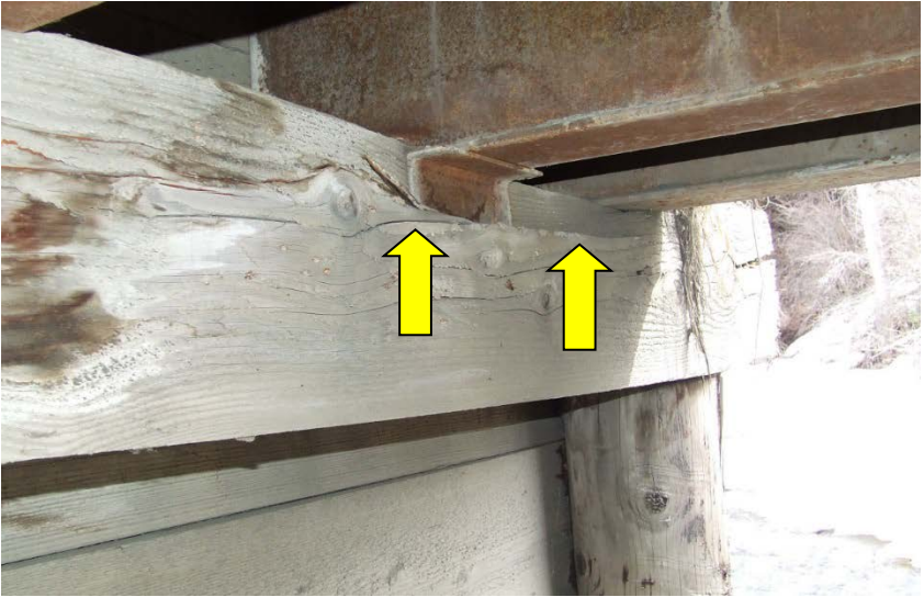
Crushing due to decay
