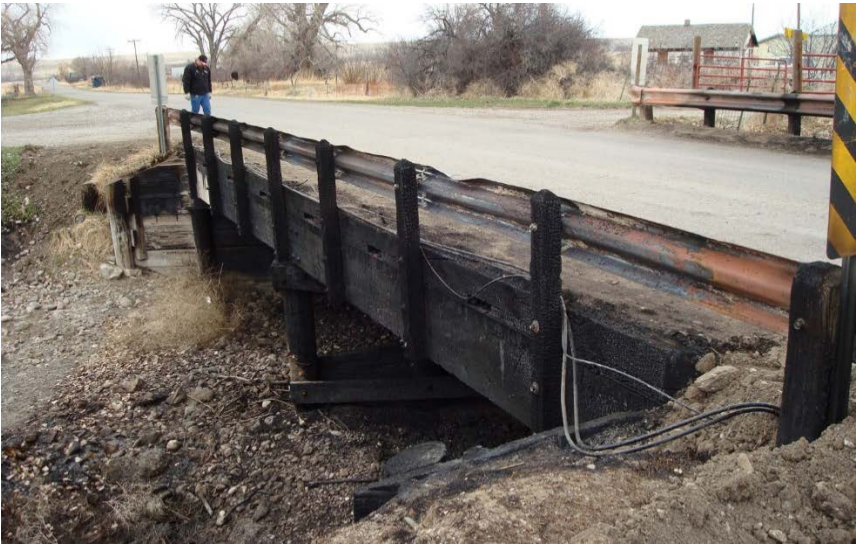
Timber bridge after a fire
