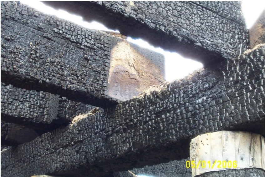
Considerable section is left on members under the char layer
