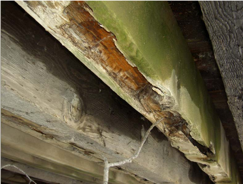
Severe decay in a girder
