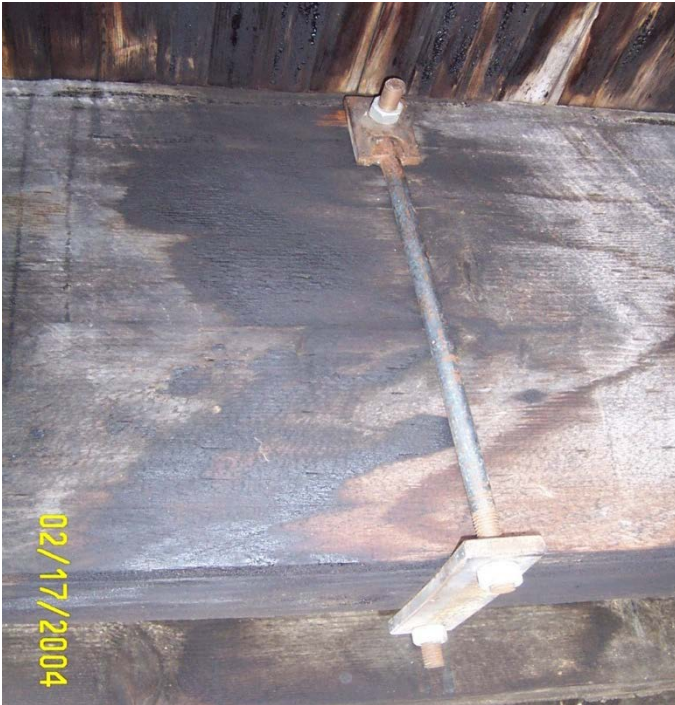
Steel hanger girder repair - single bolt and no bottom plate
