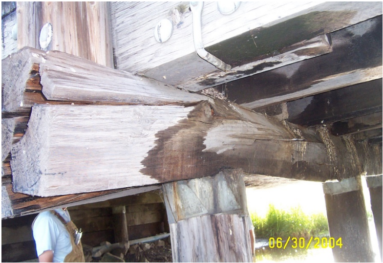
Severe crushing due to decay
