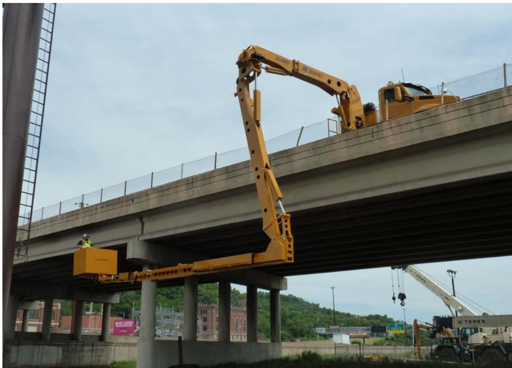
BOOM-2 AND BOOM-3 HAVE NOW BEEN OPERATED TO “OPEN” SUFFICIENTLY TO ENABLE PLATFORM TO BE POSITIONED UNDER THE BRIDGE DECK
