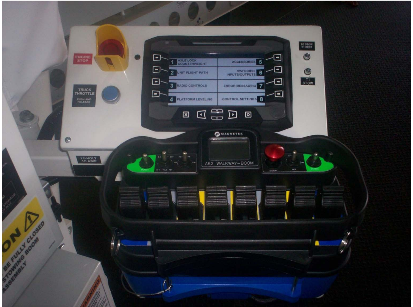
Radio control box and DP700 control at T1 Station
