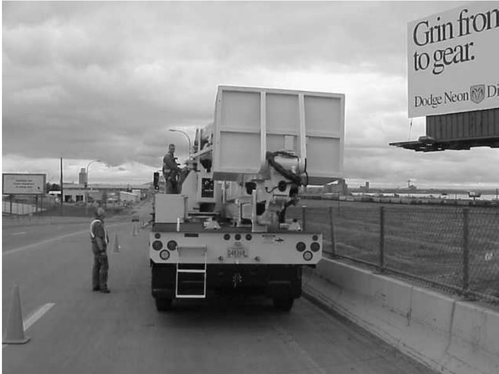
UNIT IS PARKED AT THE BRIDGE SITE, AXLE LOCKS ARE ENGAGED AND SLIDING COUNTERWEIGHT IS EXTENDED, BOOM #4 IS LOWERED SLIGHTLY
