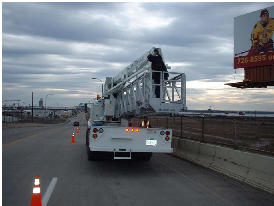
RAISE B1 TO ALLOW CLEARANCE FROM THE DECK AND ROTATE T2 CLOCKWISE AND T1 COUNTER CLOCKWISE
