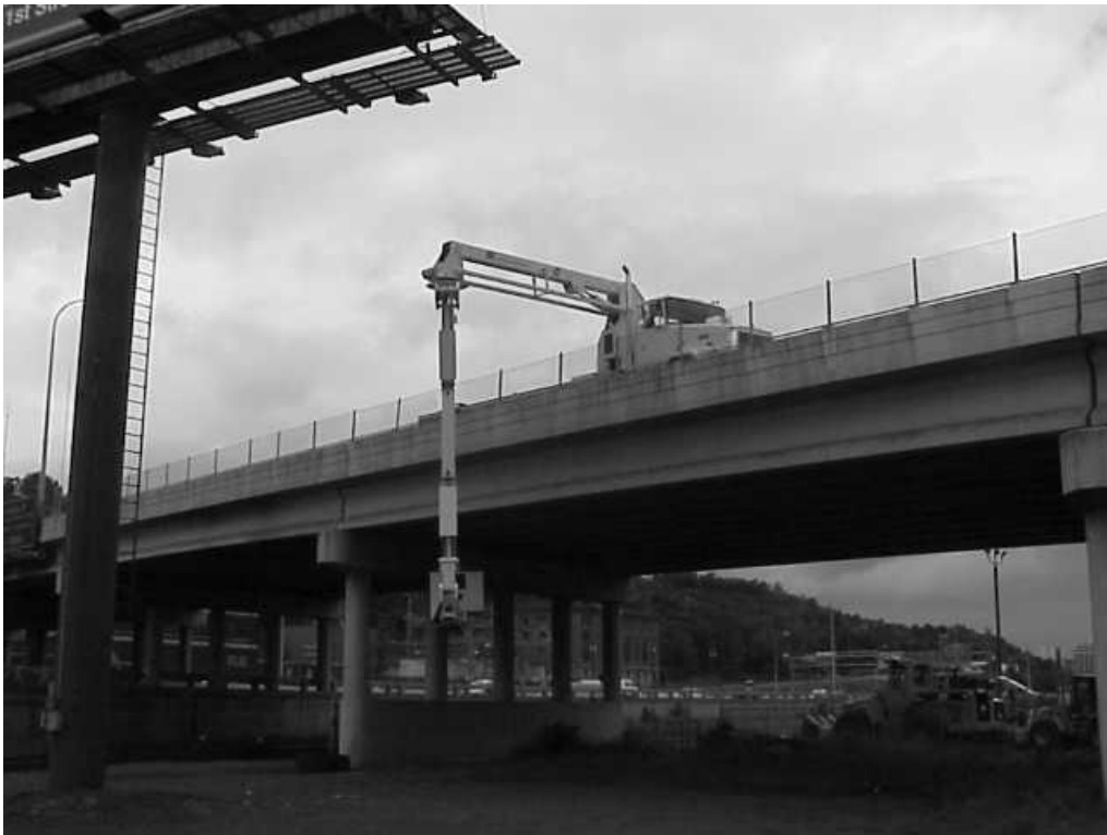
TURNTABLE #2 IS BEING ROTATED CLOCKWISE TO BRING BOOMS #3 AND #4 TO THE DESIRED POSITION UNDER THE BRIDGE
