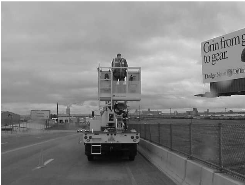
FROM THE PLATFORM AND BOOM #4 IS RAISED TO A POSITION SLIGHTLY HIGHER THAN THE BOTTOM OF BOOM THREE
