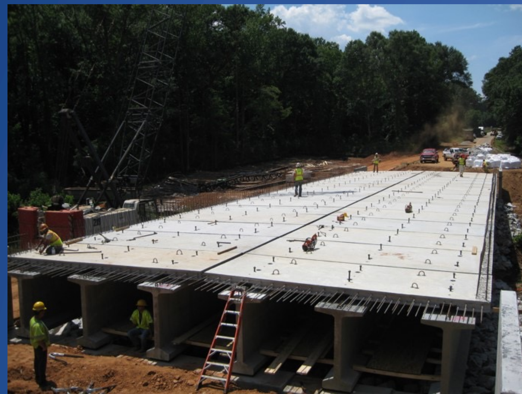
Beech Creek Bridge in Georgia Using UHPC in between Precast Deck Panels
