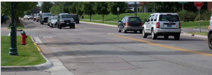
The pavement on Baker Avenue was not designed to carry heavy loads. Some rutting and cracking has been observed.
