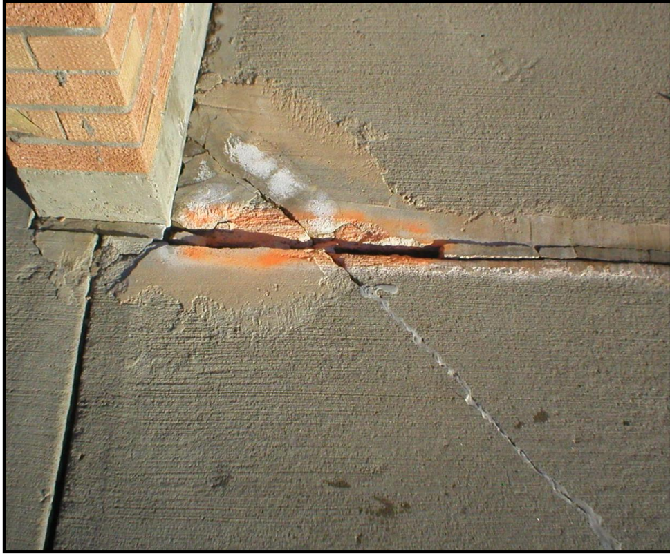
Photo 15. Cracked sidewalk at Hathaway EB site.
