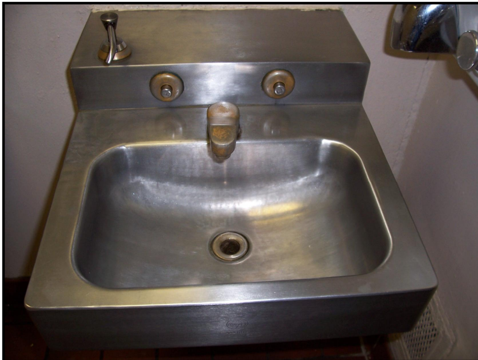
Photo 12. Rusted sink at Hysham WB site.
