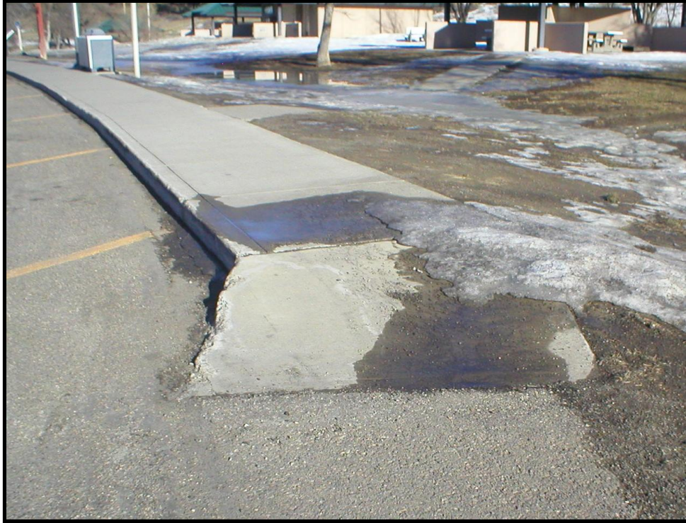
Photo 11. Crumbling ramp at Hysham EB site.
