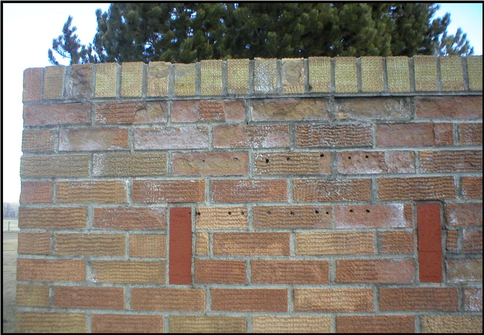
Photo 3. Crumbling brick at Greycliff WB site.
