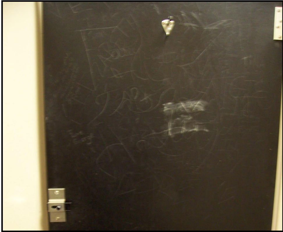
Photo 13. Graffiti on door of women's stall at Hysham WB site.
