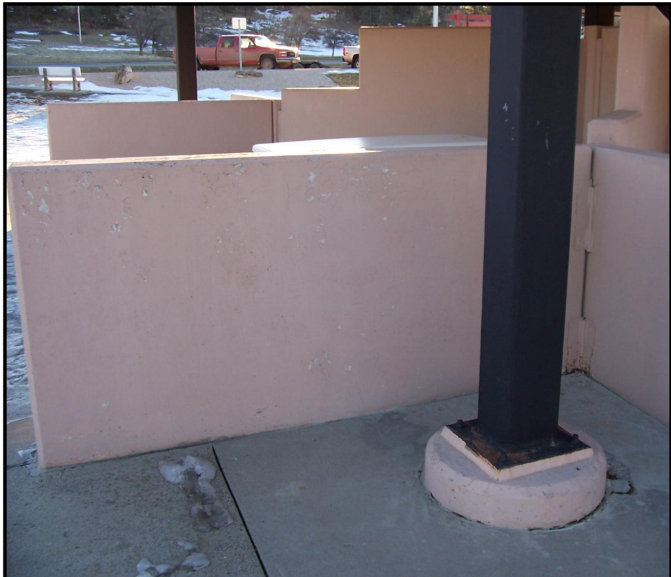
Photo 14. Chipped paint near picnic tables at Hysham WB site.
