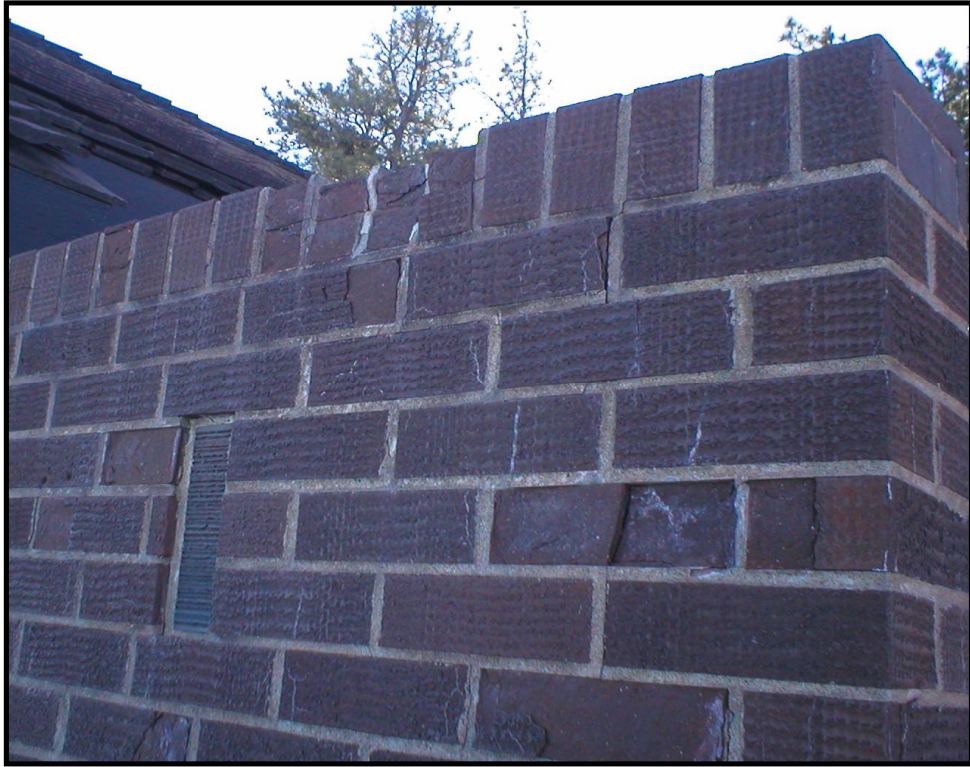
Photo 7. Crumbling brick at Custer EB site.
