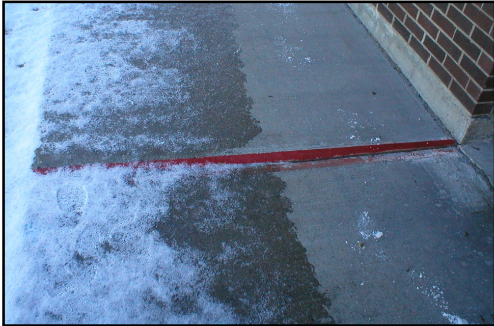
Photo 5. Uneven sidewalk at Custer EB site.
