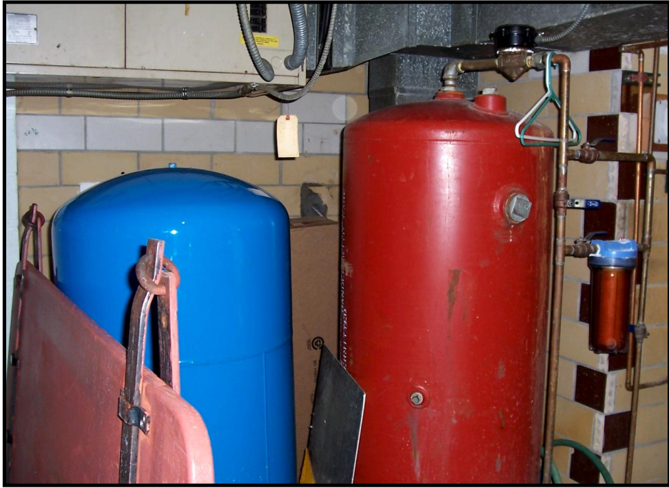
Photo 19. Pressure tanks for Custer EB.
