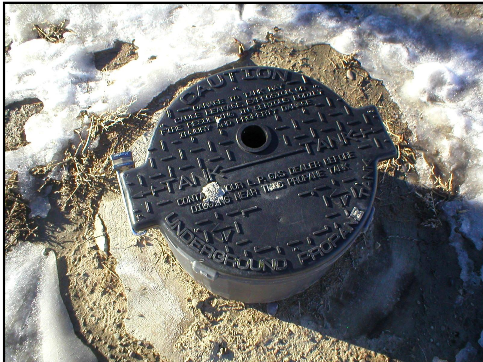
Photo 35. Underground propane tank at Hathaway EB.
