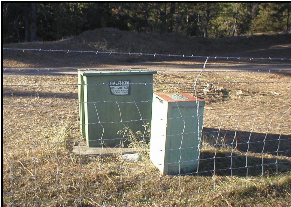
Photo 5. Power source located outside fence at Greycliff EB site.
