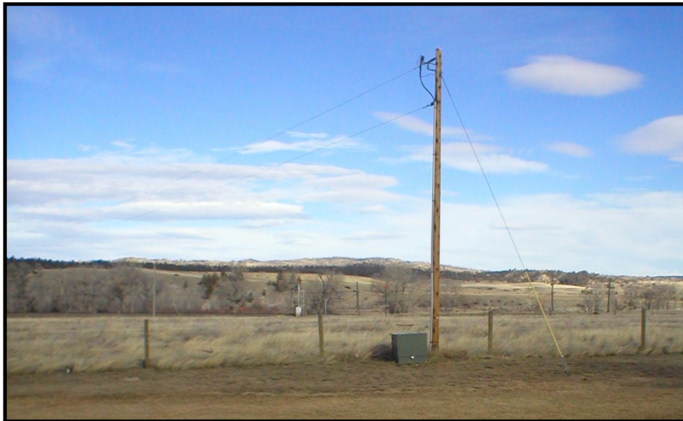
Photo 7. Power source for Greycliff WB.
