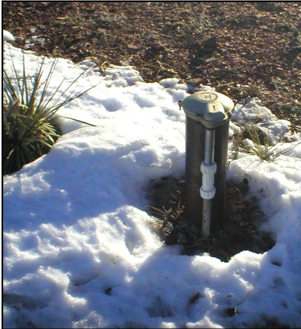
Photo 39. Well head for Hathaway EB.
