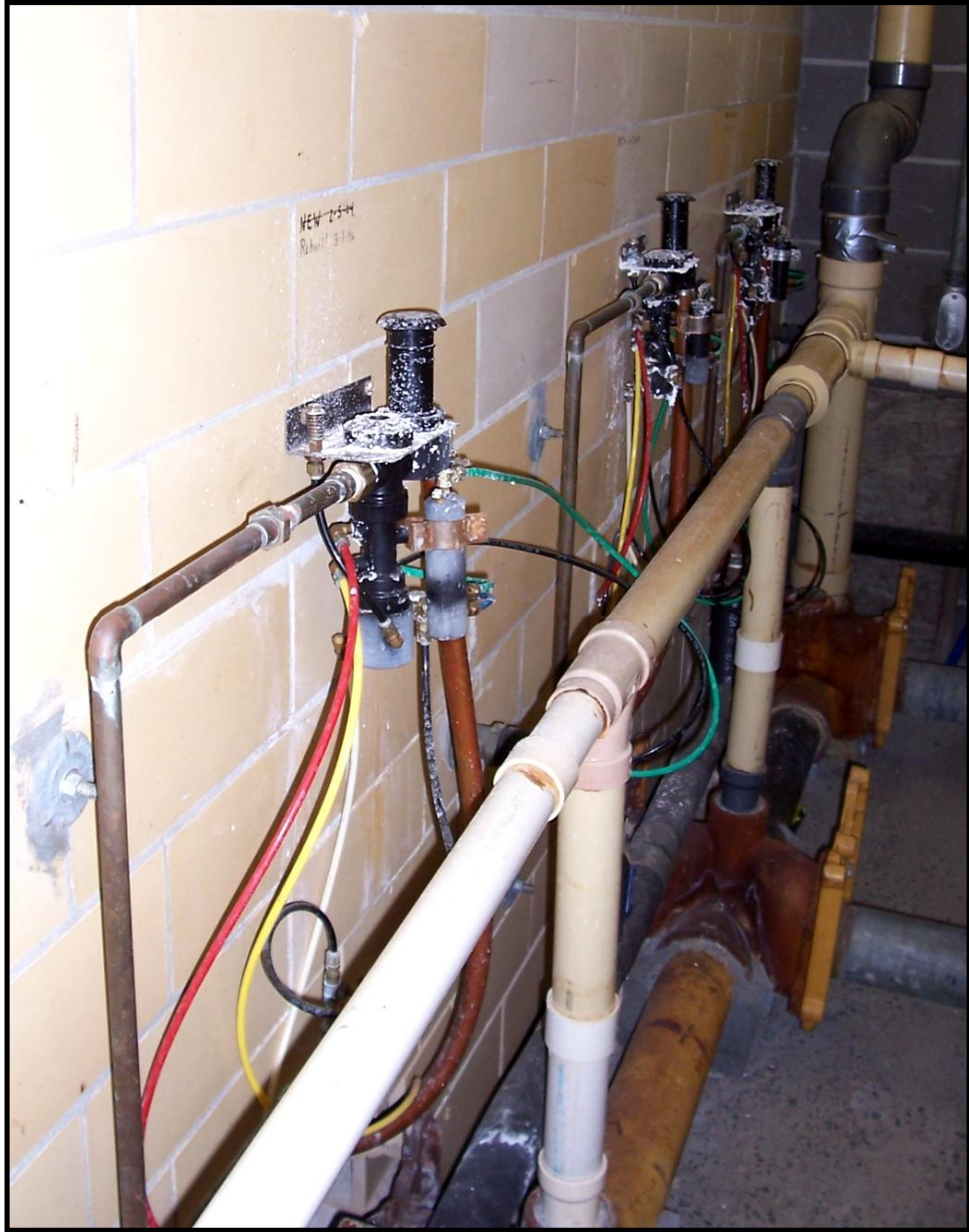
Photo 18. Air valves for toilet operation.
