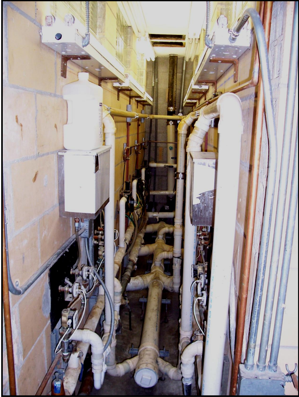
Photo 10. Water and Sewer Plumbing
