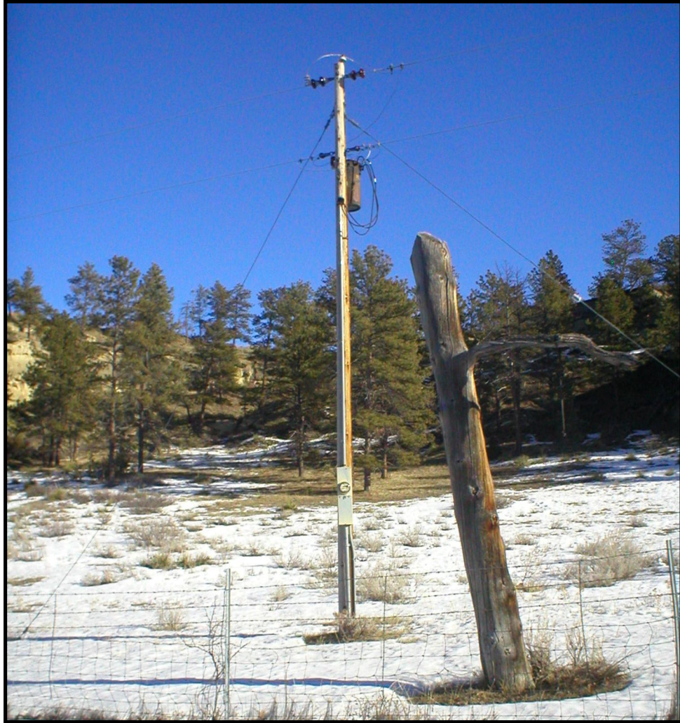
Photo 25. Power source for Hysham EB site.
