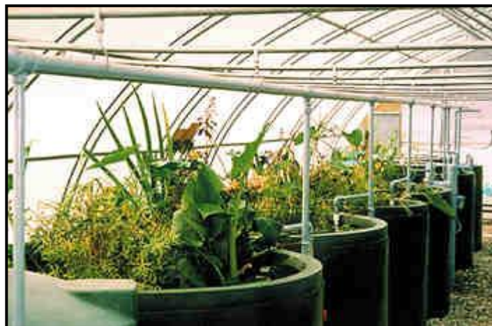
Inside the rest area's wastewater treatment system, plants and animals clean the waste from the water through a series of engineered ecosystems. (Photo by Living Technologies)
