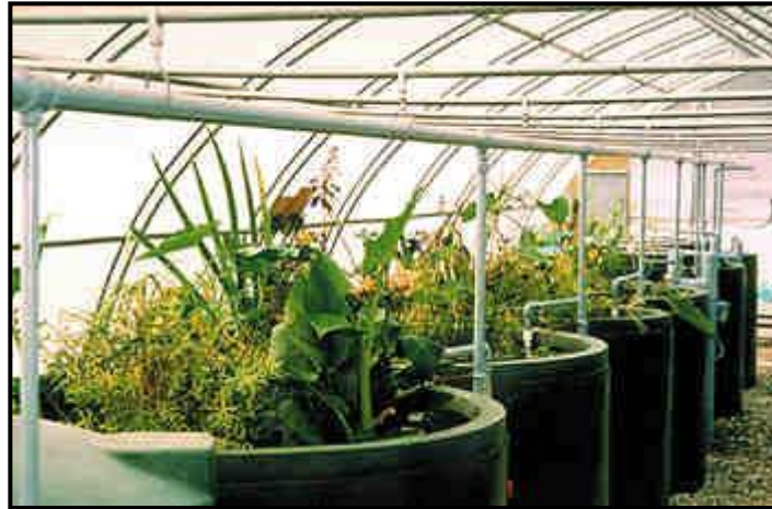
Inside the rest area's wastewater treatment system, plants and animals clean the waste from the water through a series of engineered ecosystems. (Photo by Living Technologies)
