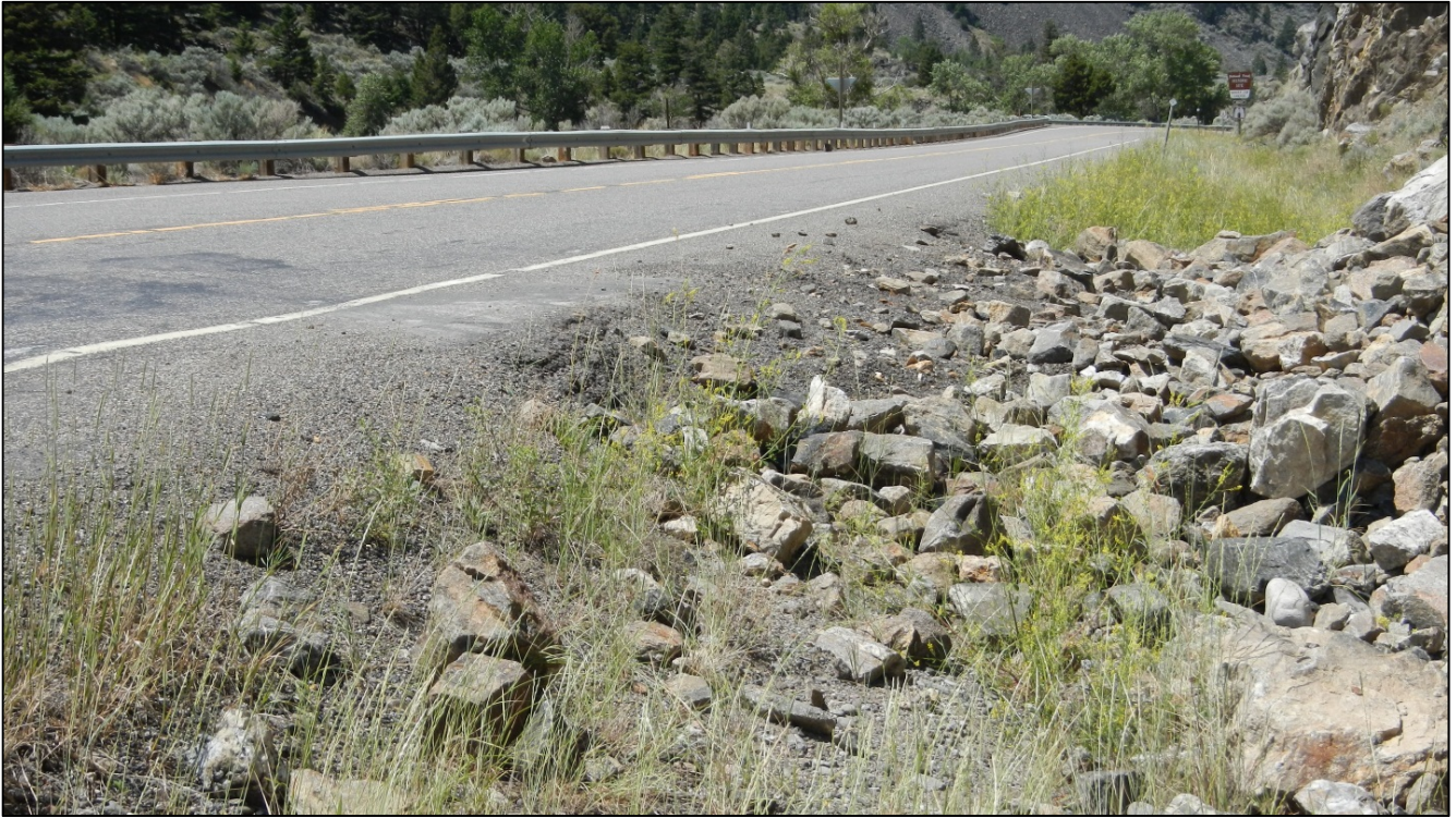
PHOTO 19: RP 13.5, LOOKING WEST (NOTE ROCKFALL ON RIGHT)
