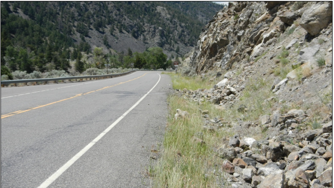
PHOTO 18: RP 13.5, LOOKING WEST (NOTE ROCKFALL ON RIGHT)
