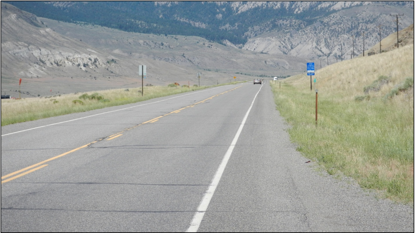
PHOTO 6: RP 2.0, US 89 NEAR THE GARDINER AIRPORT (LOOKING WEST)
