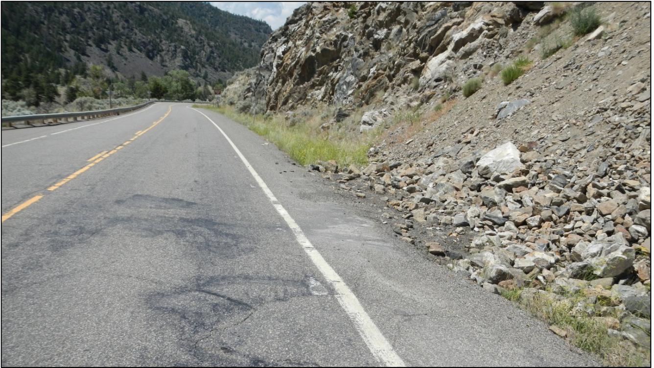
PHOTO 20: RP 13.5, LOOKING WEST (NOTE ROCKFALL ON RIGHT)
