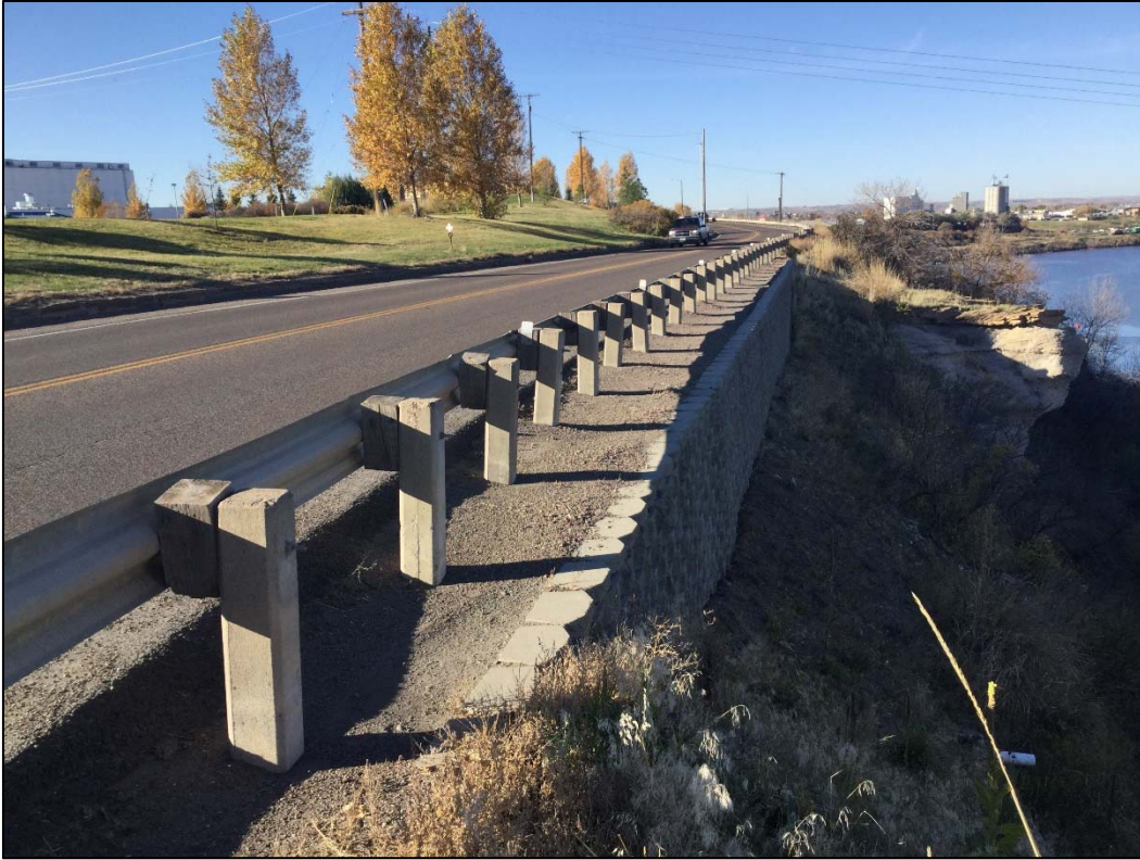
Photo 21: Looking west at the retaining wall near the Veteran's Memorial Park (RP 4.5)
