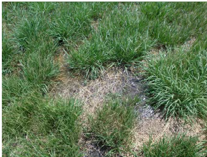
Photo 154. Segment 5, RP 527.1±, evidence of wastewater blockage at existing Vandalia Rest Area site.
